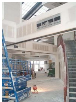
SCS Interior Lower Level
